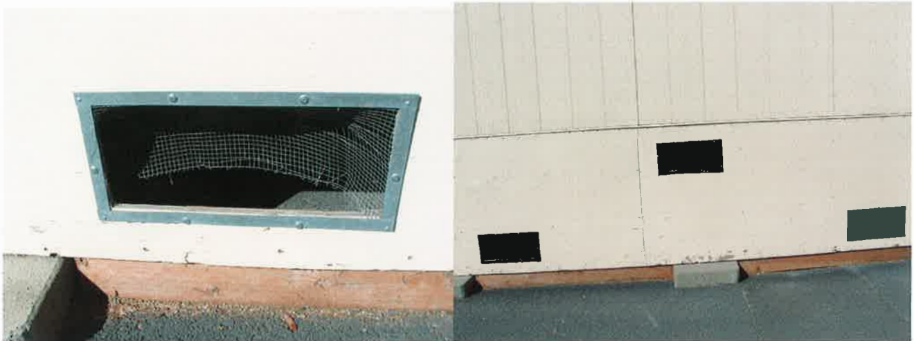
Picture taken 4-09-2013 – West Park Elementary Additional Modular Classroom Typical ventings
