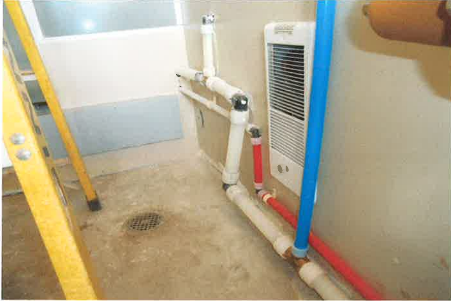
Mechanical room wall heater and electrical panels. Lowest equipment
