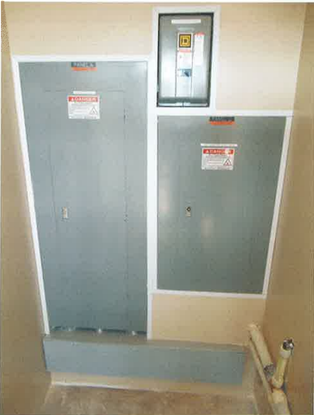
Electrical panels mechanical room concession stand access.
